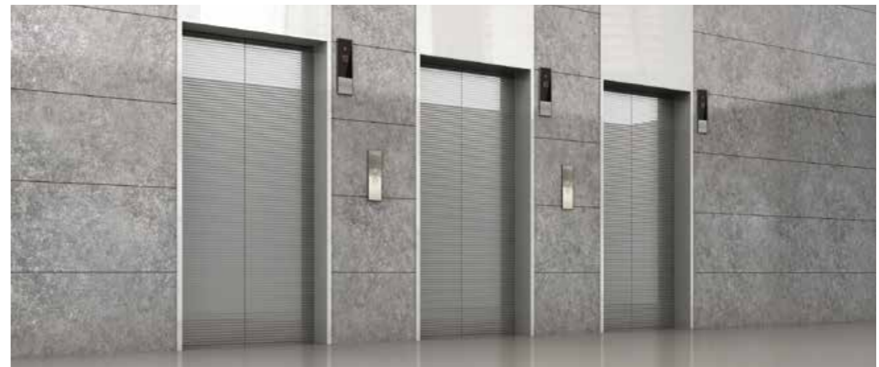
Group Supervisory Control
